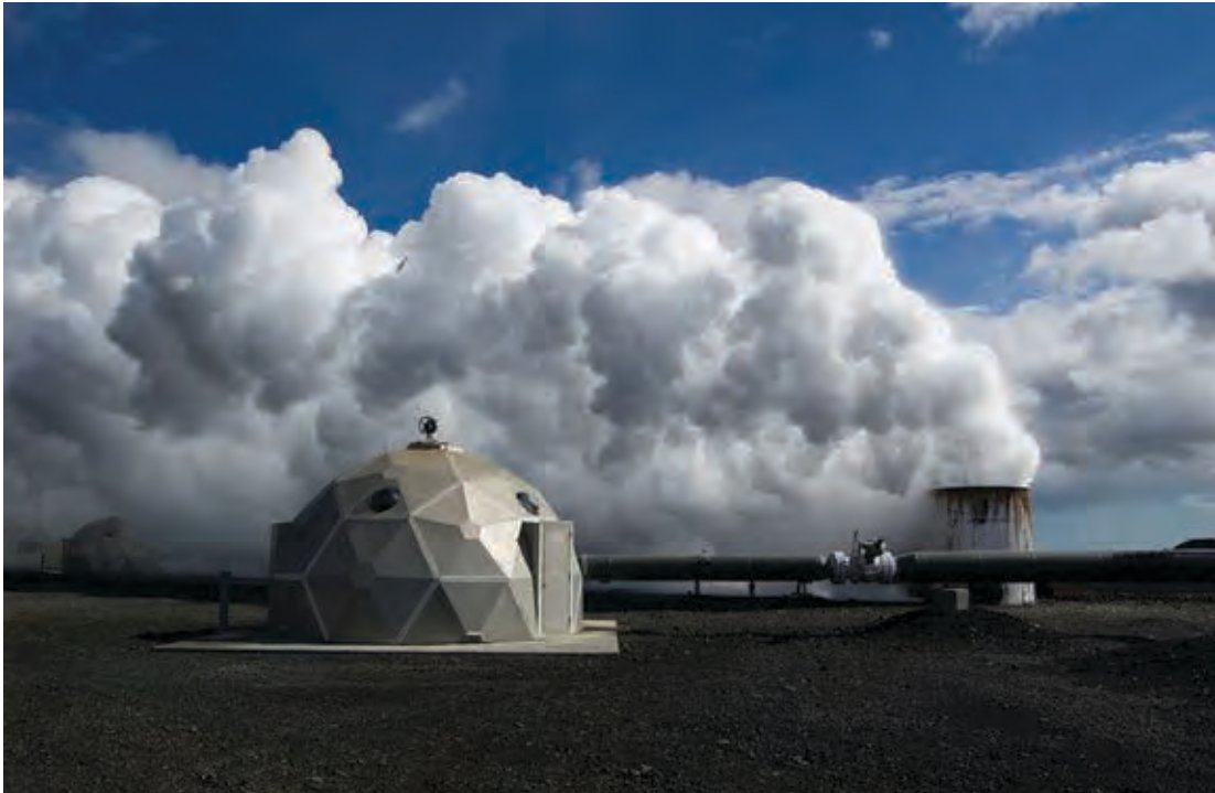
FIGURE 2.4 Geothermal Well Head and Silencer
